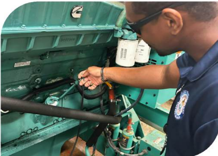
HMCI inspecting generators at one of the shelters.
