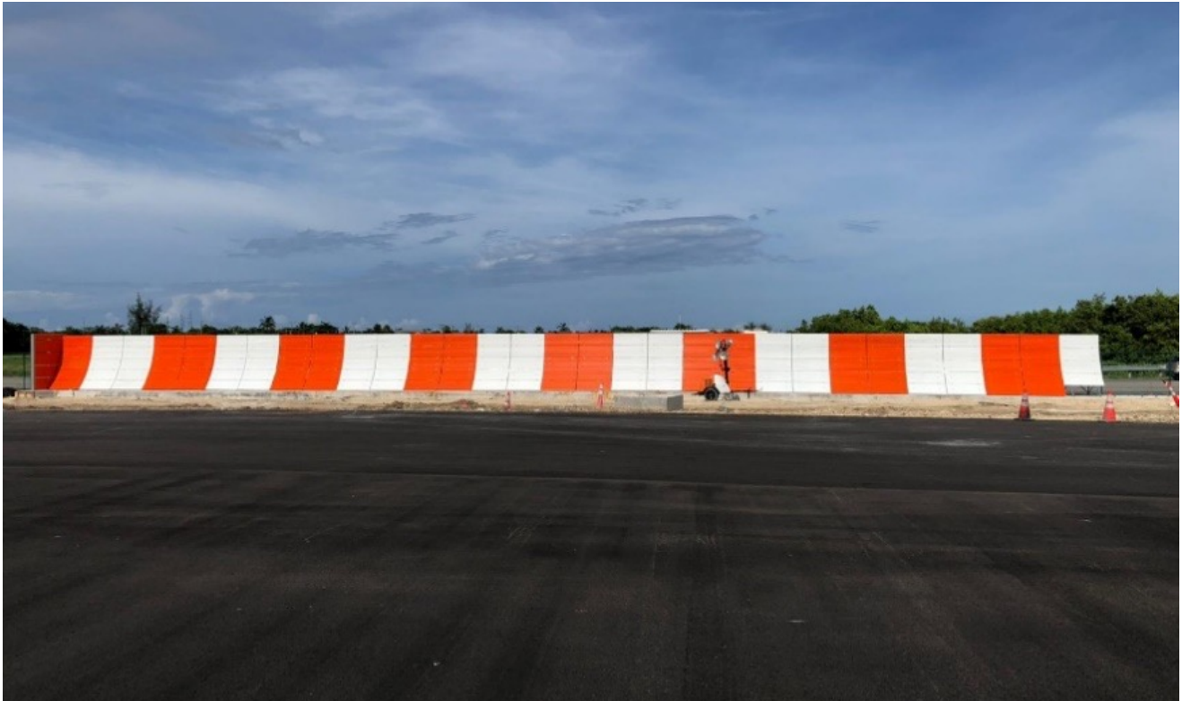
A section of the new blast deflector at Owen Roberts International Airport
