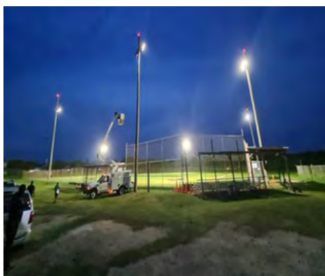
WEST BAY SOFTBALL FIELD WITH LED FLOODLIGHT
