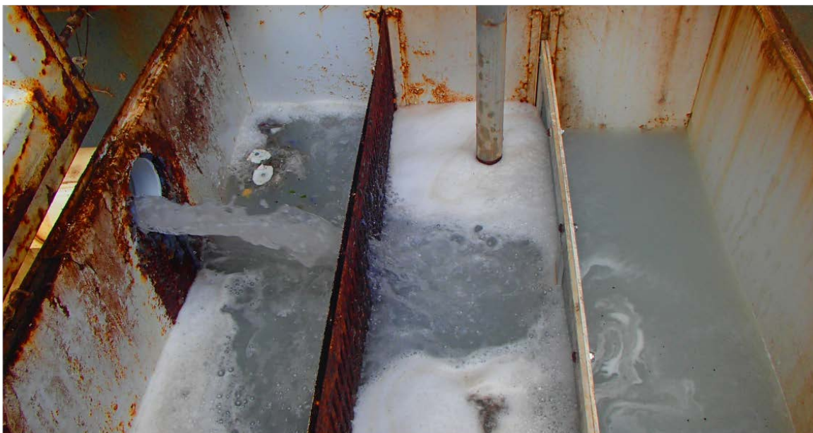
Testing at a substandard treatment plant.
