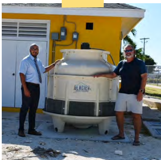
DOS Director Kurt Hyde & CIASA President Stephen Broadbelt with the newly installed Pool Chiller
