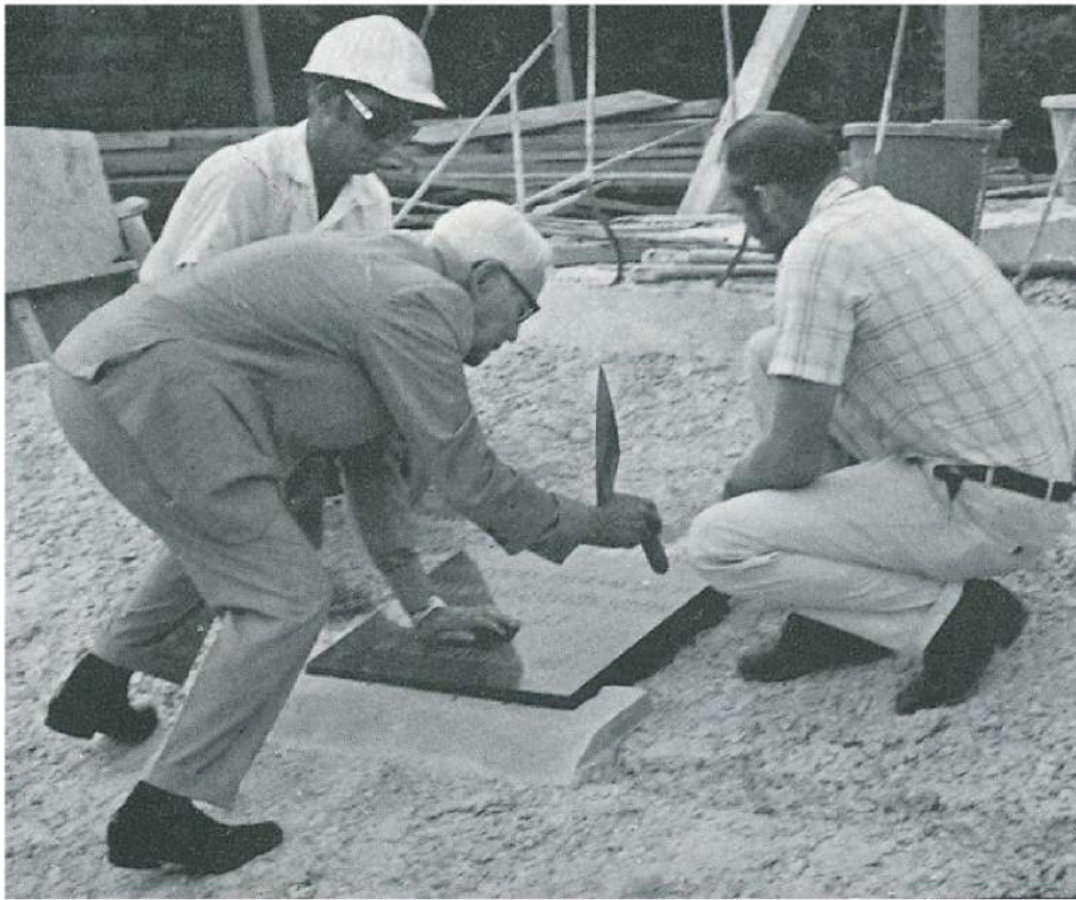
Left: Mr. David Arch of Arch Construction assists Capt. Rayal Bodden in the laying of the cornerstone, 29th September 1971. (Compass Media Ltd.)
