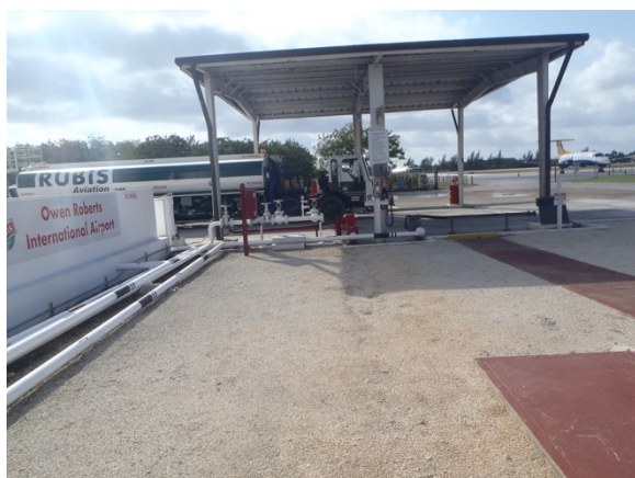
Fueling facilities at Owen Roberts International Airport in George Town
