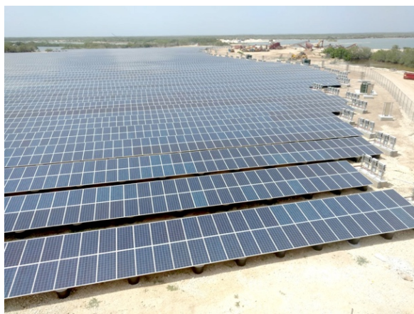
5 MW utility-scale PV solar plant in Bodden Town
