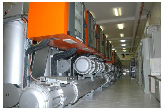
Switchgear at CUC's North Sound Substation
