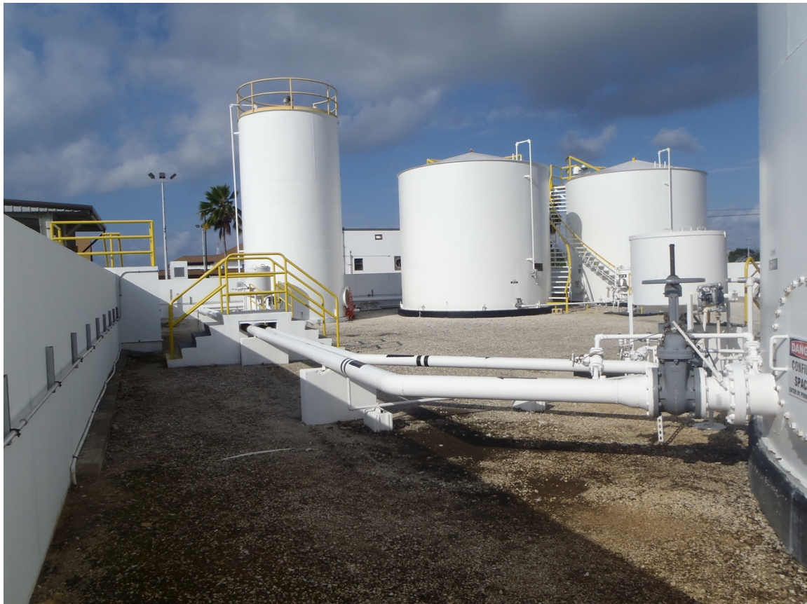
Bulk fuel handling facility in the Cayman Islands
